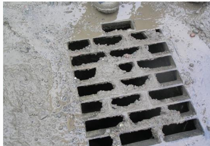
Not Adequately protected
