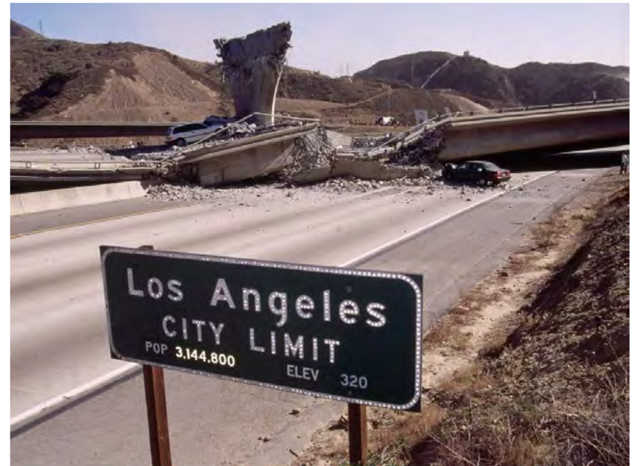
Photo: Freeway overpass collapse in 1994 Northridge Earthquake
